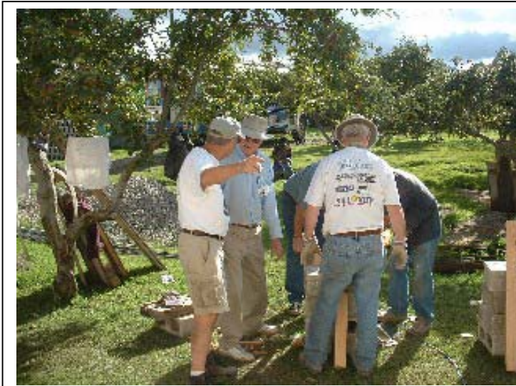
Building Beds – The construction team at Comanchaj built the first of two bunk beds. The contractors helping with construction were sleeping on the floor until our team built them a bed. (The three team members in front, left-to-right, are Jerry Malone, Robert Gross, and Terry Baughn.)
