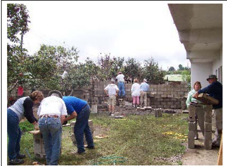
The team is building a wall around the Salud y Paz compound.
