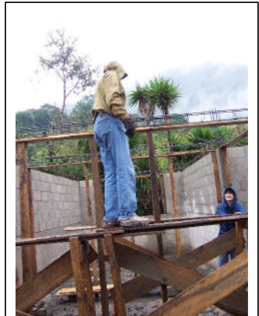
Mark Jacobson putting up forms for the concrete to be poured later
