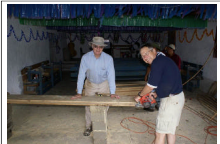
Robert Gross and Jerry Malone at the work site, cutting boards for forms
